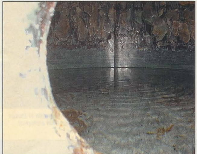
Following three months of electronic water conditioning of the domestic-hot-water services, the downtime to remove scale from this 1500 litre calorifier was around six hours.
